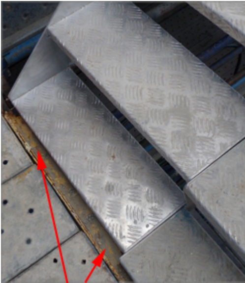
Photograph 4 – Excessive gap on transom (indicated by arrows).
