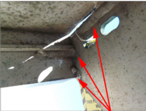
Photograph 3 – Underside view of failed module welds (shown by arrows).
