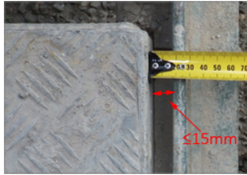
Photograph 5 –The gap between the vertical face of the transom and end of stairs should not exceed 15 mm (unless otherwise specified by scaffolding manufacturer).
