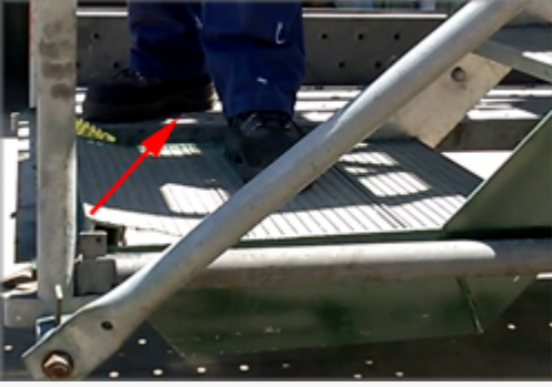
Photograph 2 – Aluminium deck peeled away (as indicated by arrow) when a worker stepped onto it and the stairs dropped.
