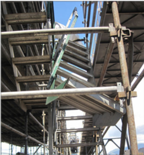
Photograph 1 - Single width aluminium stair module after one incident
