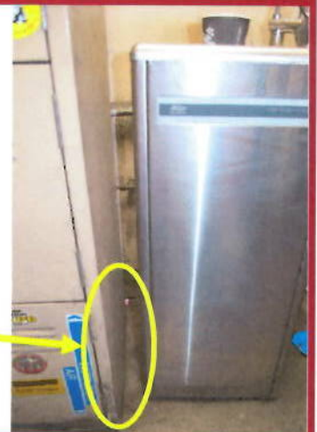
Electrical lead was positioned under the metallic locker
