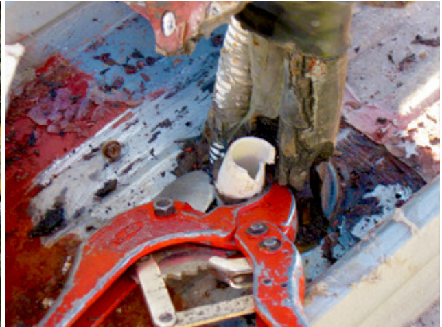
Photo 2: Electrical conduit next to drain pipe.
