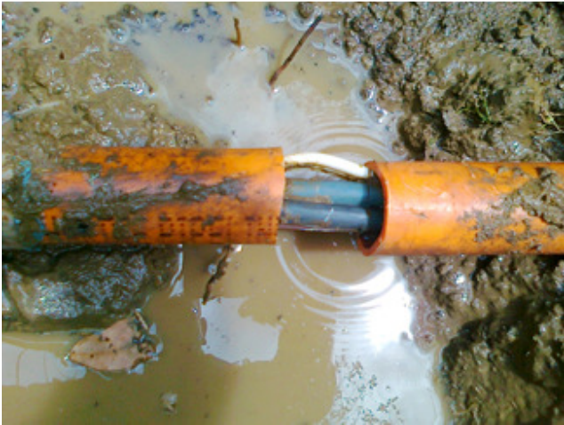
Photo 1: Separate circuits within the same conduit.
