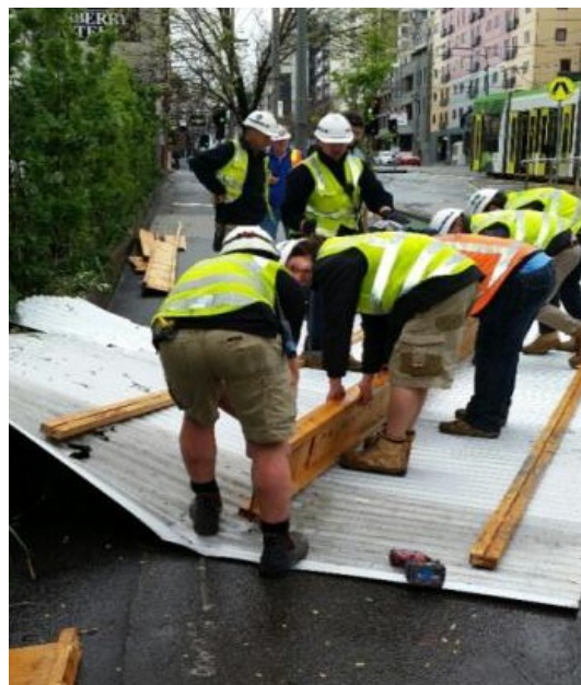
A temporary site awning blew into an adjacent street
