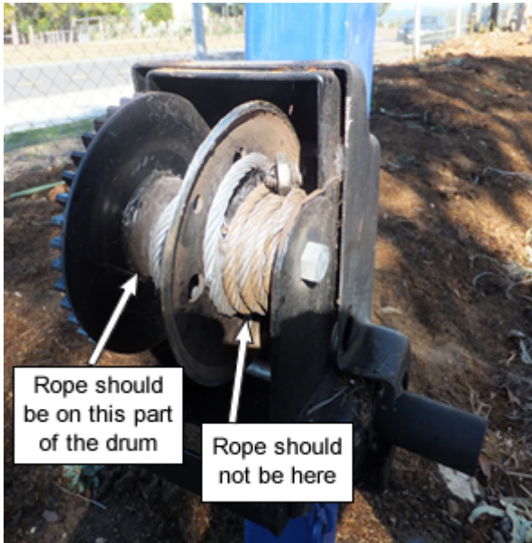
Photograph 2 - Wire rope has wound off winch drum and onto winch shaft on the right of the drum.
