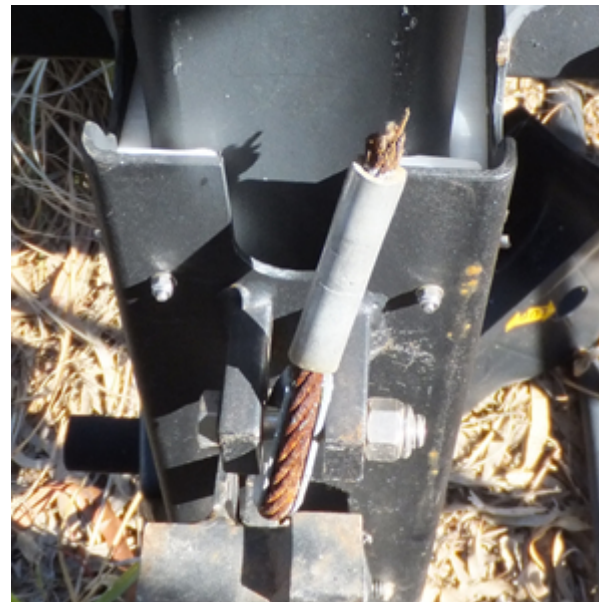
Photograph 5 - Broken hoist wire (caused by corrosion and possibly over-winding) on a winch type sign.
