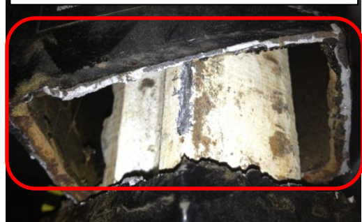
Failed section of the Support Stand
